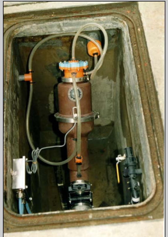
Interface Valve in bespoke chambers
